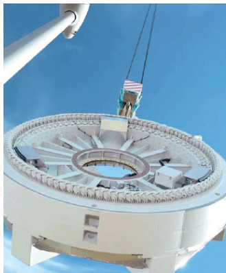
Figure 6: The assembled generator is lifted to the top of the wind turbine tower. It weighs 30 tonnes, and about a third of that weight is copper. (Courtesy of Enercon.)
